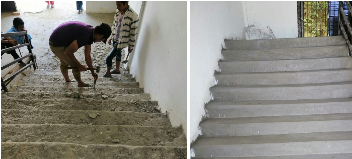
Fig: Improved construction work of school after the monitoring (The materials used on the stairs were of not good quality so reconstruction monitoring group in coordination with advocacy group made the contractors to make it with good quality)
