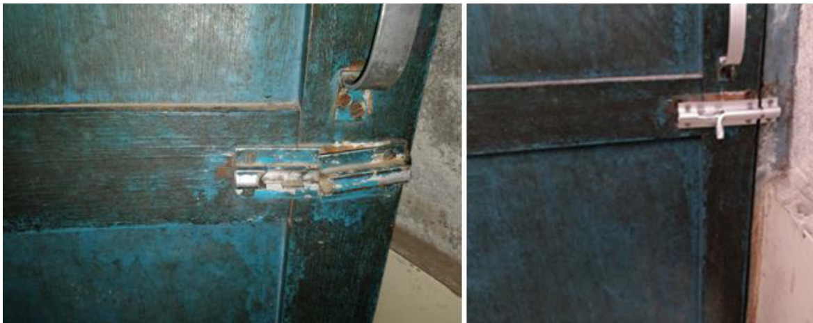
Fig: The lock of girls' toilet was not repaired by school since 6 months, Reconstruction monitoring group of integrity club led to repair the lock
