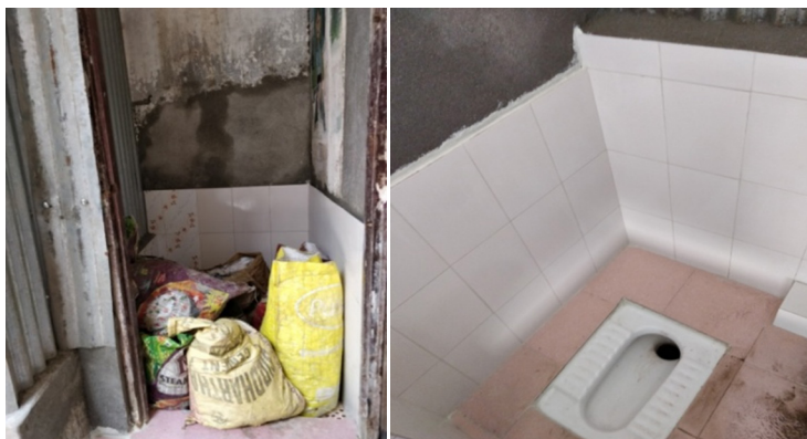
Fig: The toilet of the school that used to be a dustbin and store was transformed into the proper toilet in a usable condition- led by WASH group of Integrity club
